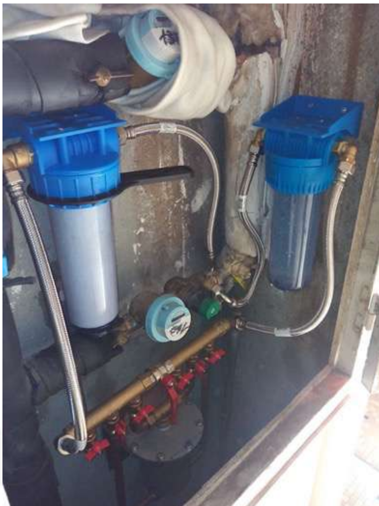
(In a narrow technical duct)
